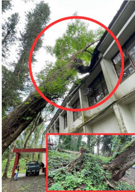
Figure 14. Tree Failure Located in Florencio Tamesis Hall Showing Uplifted Roots and Structural Damage
